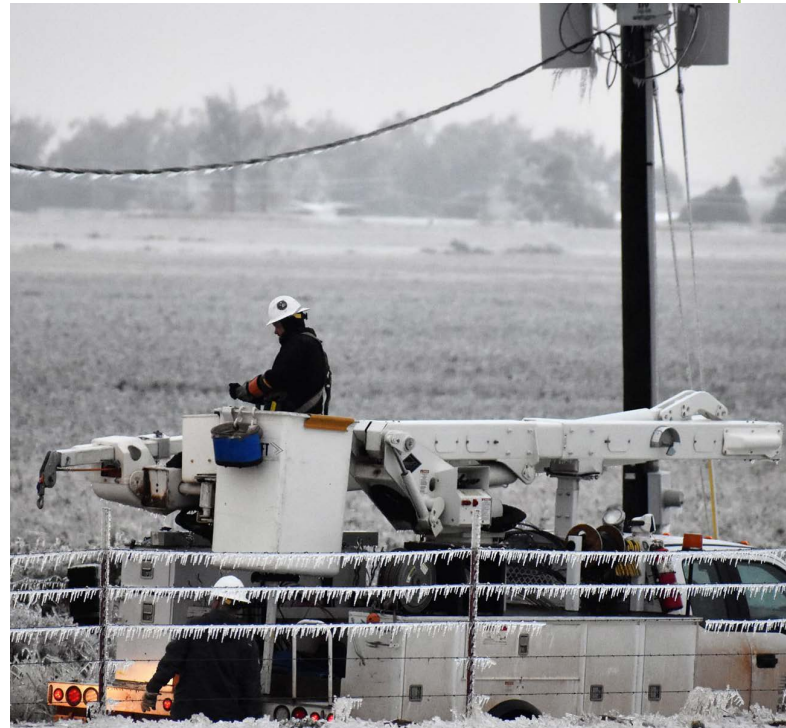
Pictured: Crews restoring power during the 2020 ice storm. Photo courtesy of Whitney Huff.
